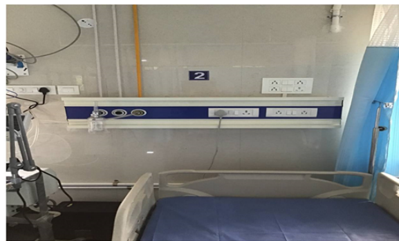
figure 2: Bed Head panels which included a central suction port, two oxygen ports and four electrical points, were placed in all wards over each beds
