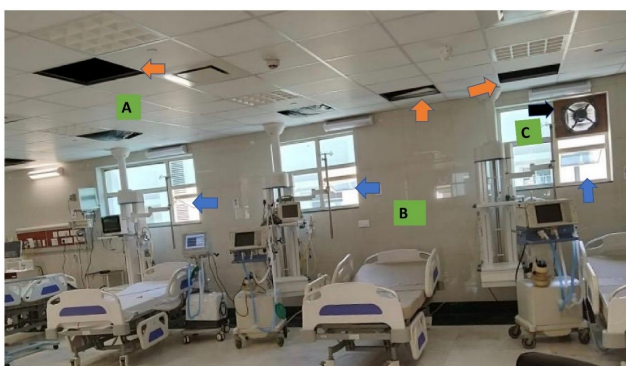
FIGURE 1: (A) Sealing of recirculation duct, (B) Opening of windows, (C) Activation of exhaust fan
